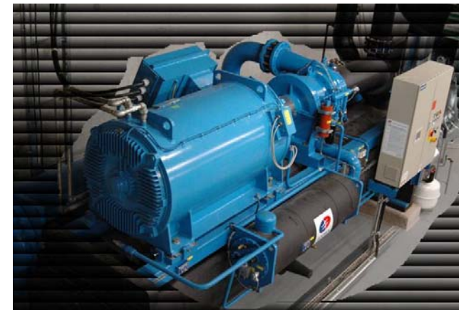
AXIMA Refrigeration Climespace Tokyo, 2005
