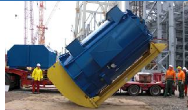
Main cooling water pump motor with tilting device
