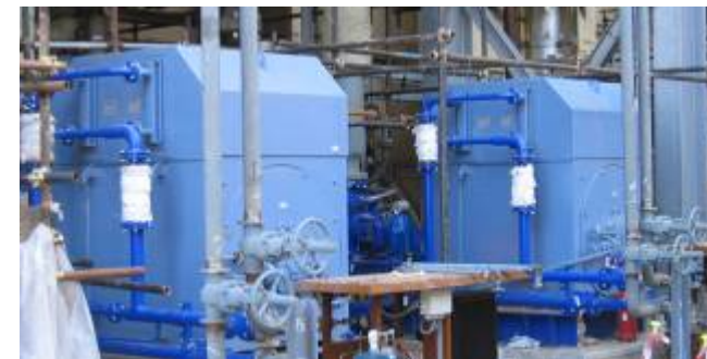
Variable-speed regulated boiler feed water pump motor / Termoli power plant, Italy
