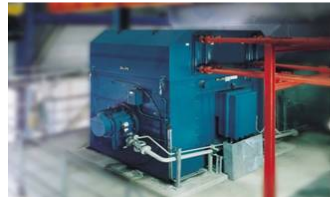
ID Fan Motor Schwarze Pumpe Power Plant, Germany
